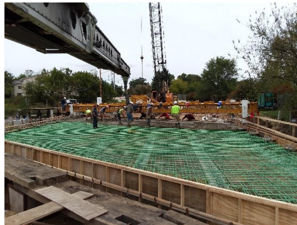
Bridge deck pour in progress – Fri. 9-28-18 Steel reinforcing for deck is epoxy coated to prevent corrosion and extend the useful life of the structure.
